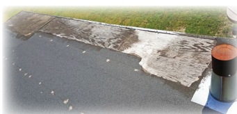
Above: The roof of the caboose is in great disrepair.
